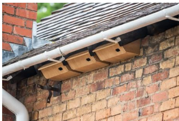
LSG boxes installed in New Street
